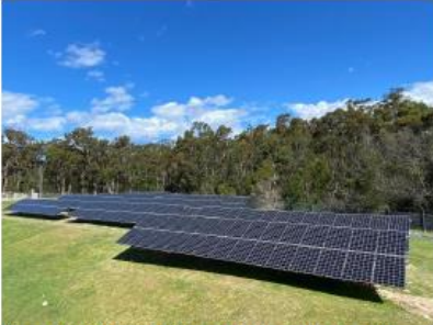
Vincentia WWTP 95 kW ground-mounted solar PV array
