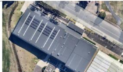
A 60kW solar PV system installed at the Shoalhaven Indoor Sports Centre in late 2021
